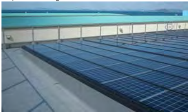
Solar panels on the roof of Matsuyama Factory No.3
