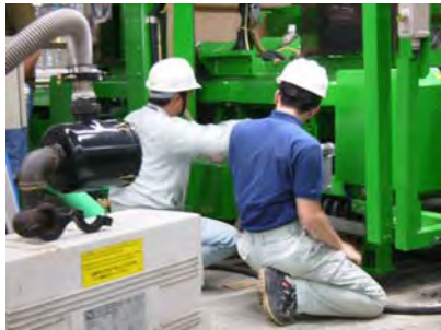
Staffs are maintaining equipment at a customer's site
