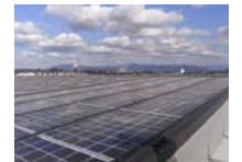
PV systems on the roof of Matsuyama factory
