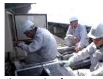
Inspection service for power plants
