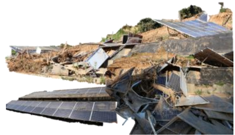
Panels damaged by a disaster in 2018 Photo by PVeye
