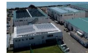
Solar power system of approx. 630 kW for in-house power consumption and electric power sales installed on the rooftop of Matsuyama Factory. (Equivalent to about 180 residential solar power systems.)
